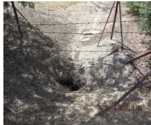
05/12/2014 (NA0017U07 LM:13.838) : Drop-inlet on LS toe.
