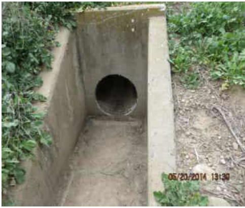
05/20/2014 (NA0017U08 LM:14.324) : Headwall at LS toe.
