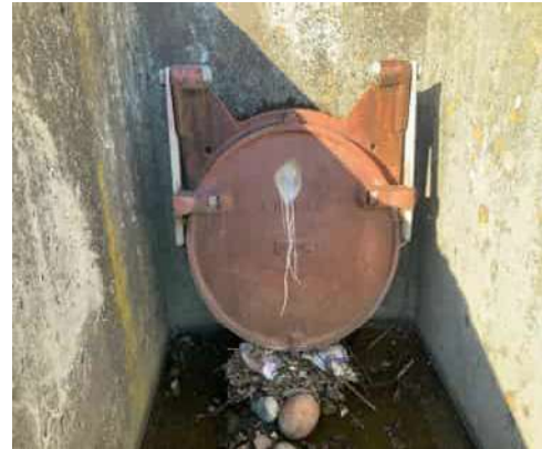
02/26/2021 (NA0017U07 LM:13.838) : WS view: WS flapgate.
