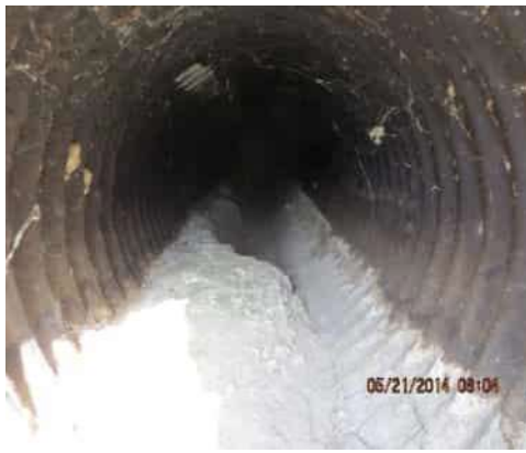
05/21/2014 (NA0017U08 LM:14.306) : Inside pipe at LS toe. Note silt buildup.
