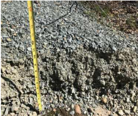
02/23/2021 (NA0017U08 LM:14.324) : LS View: Accumulation of gravel at LS toe.
