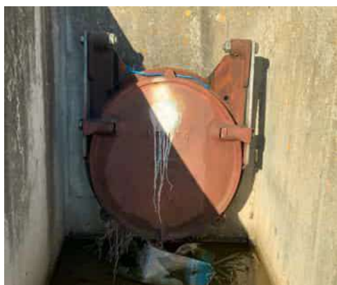
02/26/2021 (NA0017U07 LM:13.819) : WS view: WS flapgate.
