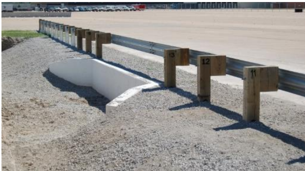
GUARDRAIL MGS (Midwest Guardrail System)
