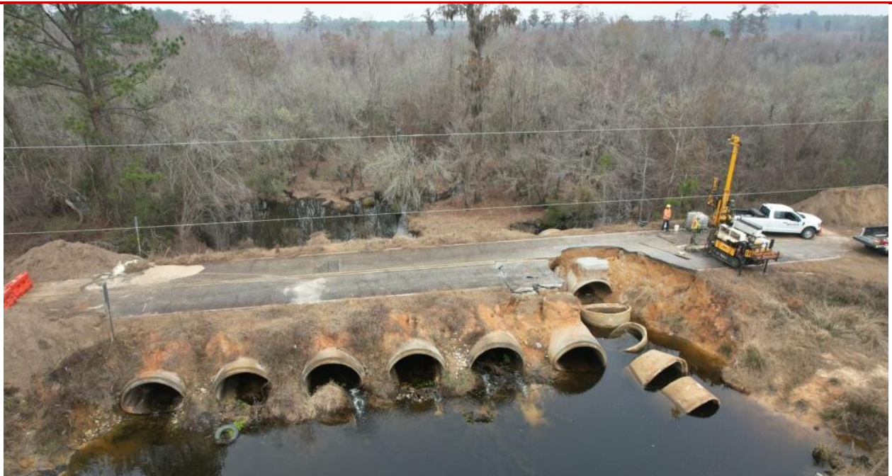
Deteriorated culvert pipes discharging into Little Lotts Creek
