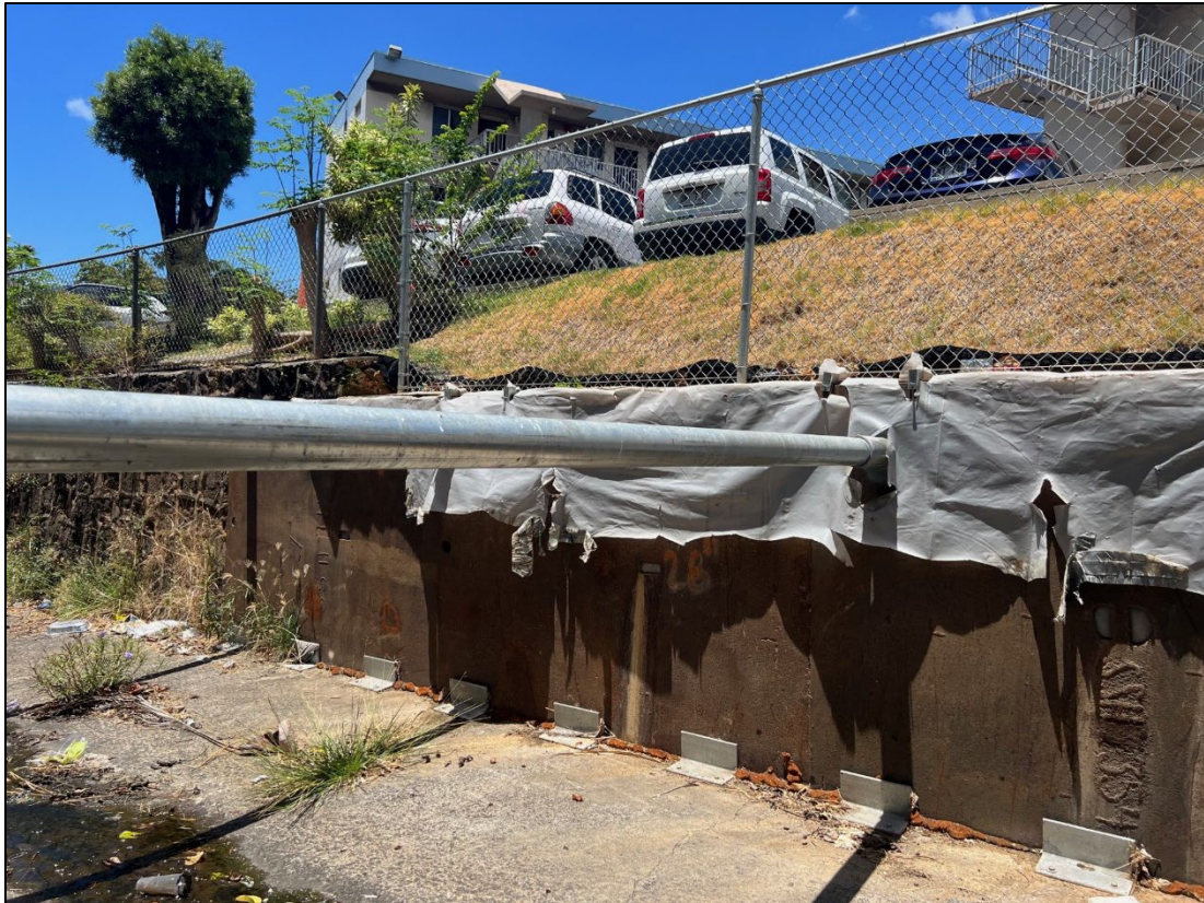
Figure 4. Screw jack braces and cleats hold metal plates where the channel walls have collapsed.
