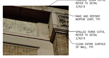
4 CRACKED TERRA COTTA SCALE: NOT TO SCALE REF: A211
