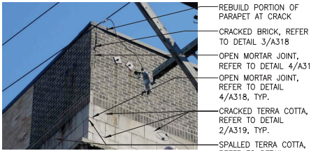
3 DAMAGED PARAPET SCALE: NOT TO SCALE REF: A309
