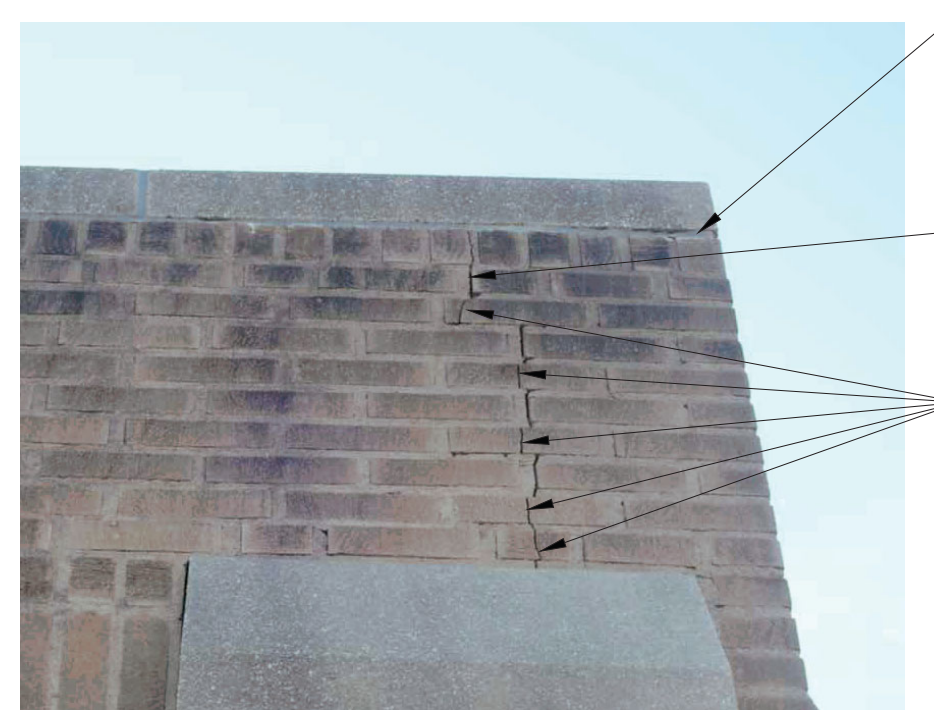
10 A409 CRACKED BRICK SCALE: NOT TO SCALE REF: A407
