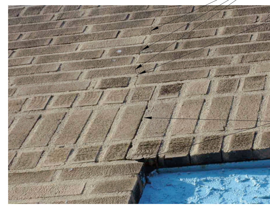
13 A409 CRACKED MORTAR JOINT SCALE: NOT TO SCALE REF: A407
