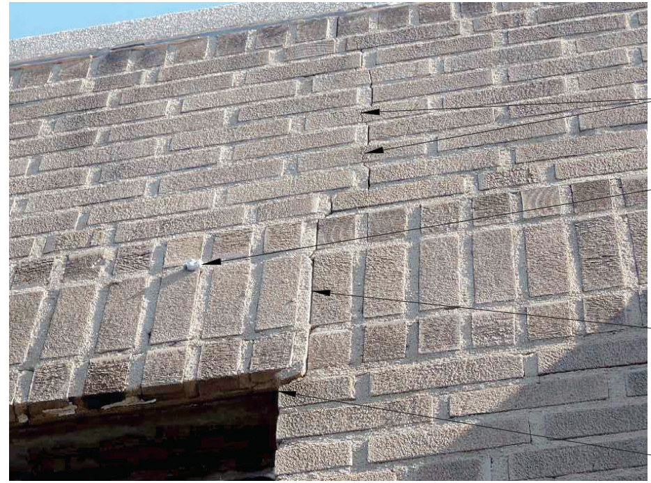
7 A410 DAMAGED LINTEL SCALE: NOT TO SCALE REF: A407
