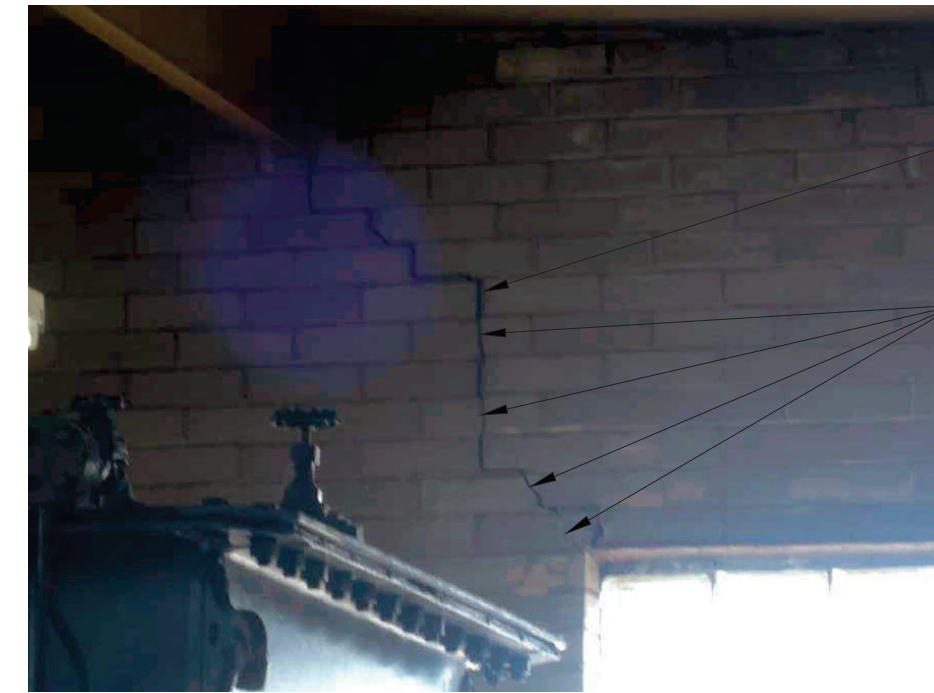
1 A409 CRACKED BRICK SCALE: NOT TO SCALE REF: A403
