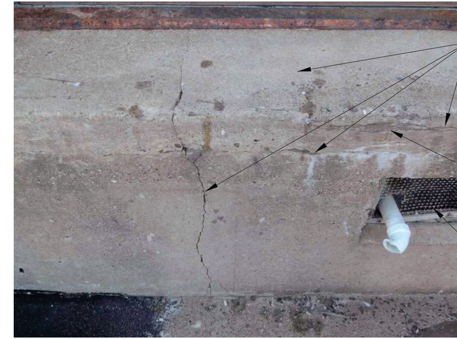
5 A409 CRACKED FOUNDATION SCALE: NOT TO SCALE REF: A407
