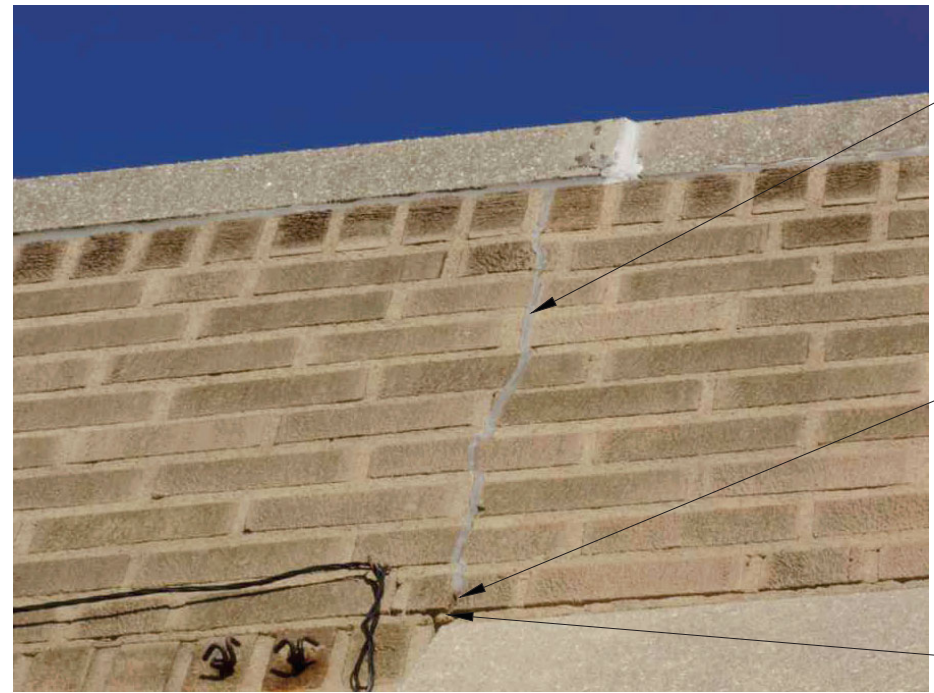
3 A410 MORTAR CRACK SCALE: NOT TO SCALE REF: A407
