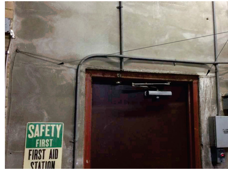
2 A409 DAMAGED WALL SCALE: NOT TO SCALE REF: A403
