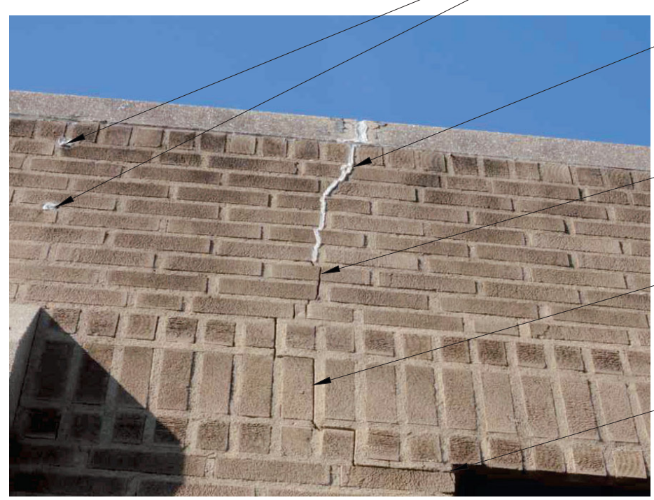
11 A409 CRACKED BRICK SCALE: NOT TO SCALE REF: A407
