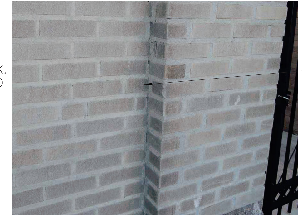
8 A409 CRACKED MORTAR JOINT SCALE: NOT TO SCALE REF: A407
