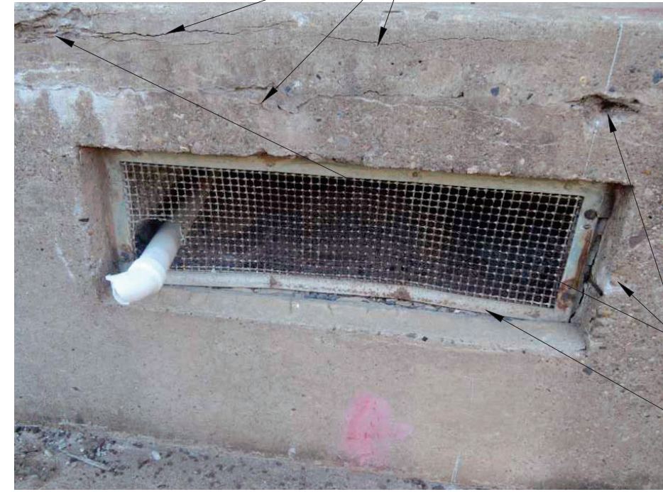
6 A409 CRACKED FOUNDATION SCALE: NOT TO SCALE REF: A407
