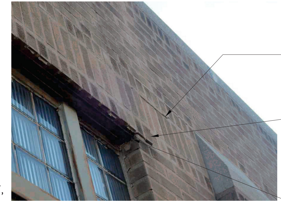
4 A410 DAMAGED LINTEL SCALE: NOT TO SCALE REF: A407
