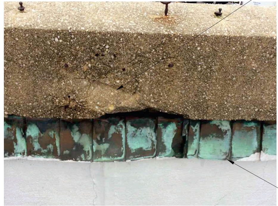
3 A409 DAMAGED COPING SCALE: NOT TO SCALE REF: A404
