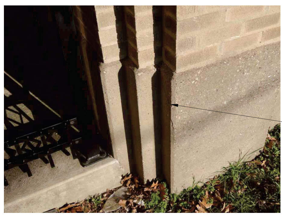
15 A409 CRACKED FOUNDATION SCALE: NOT TO SCALE REF: A407
