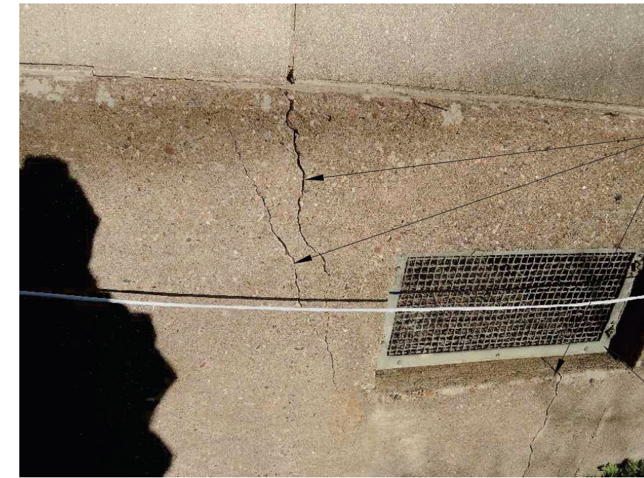
1 A410 CRACKED FOUNDATION SCALE: NOT TO SCALE REF: A407
