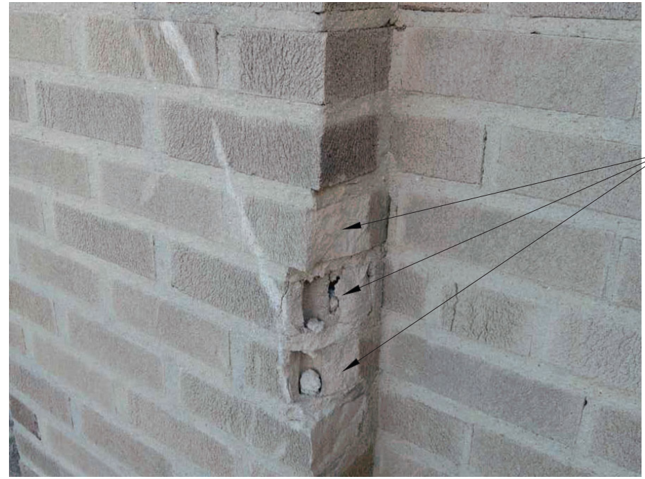
7 A409 DAMAGED BRICK SCALE: NOT TO SCALE REF: A407
