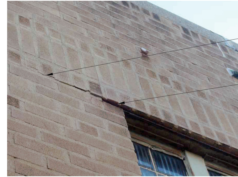
5 A410 DAMAGED LINTEL SCALE: NOT TO SCALE REF: A407
