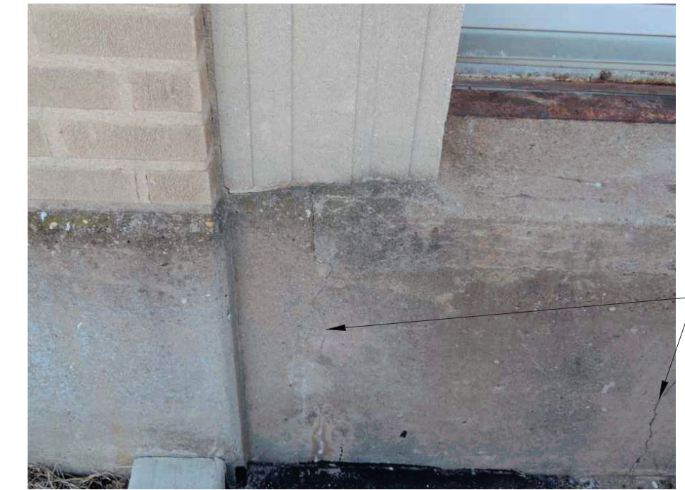
4 A409 CRACKED FOUNDATION SCALE: NOT TO SCALE REF: A407
