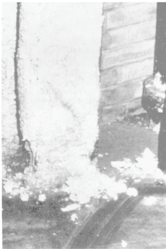
ACM which is in poor physical condition. Under a proper operations and maintenance program, corrective action would normally prevent deterioration of the insulation.
